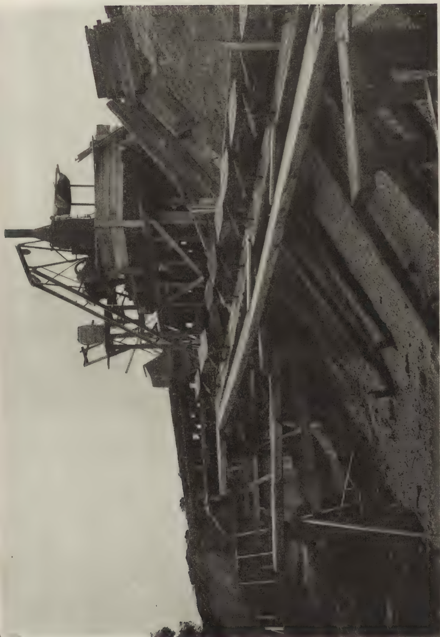
Fig. 19.—View showing method of handling the concrete materials in constructing railroad bridge abutments.
